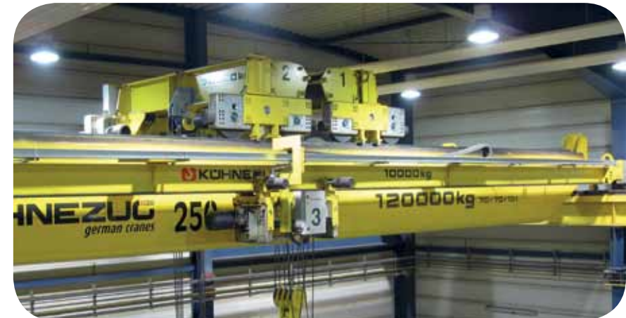
2 x 70 t + 10 t / span 18,8 m / HOL 13,5 m / steam boiler
