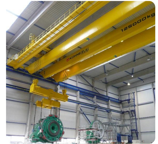
KÜHNEZUG – Double Girder Crane with 125 t Capacity.
